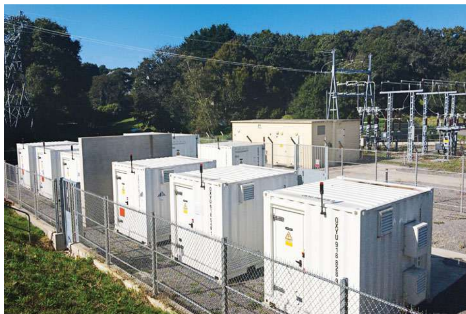
Packs, large storage areas for electric batteries.
